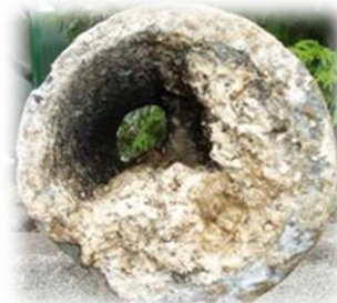
Sewer line clogged with grease
